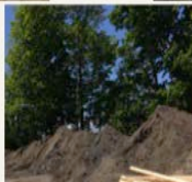
Fill for the salt ponds – oh what a difference it will make!
